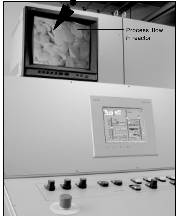
Measuring and control station in control room can be up to 1000 meters outside the Ex hazard zone.
